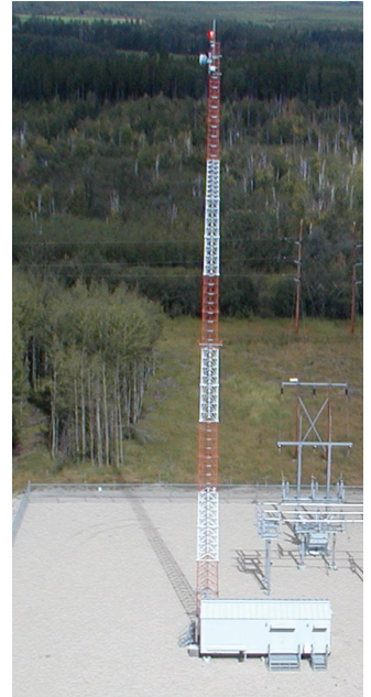
Typical self-supporting telecommunications tower.
