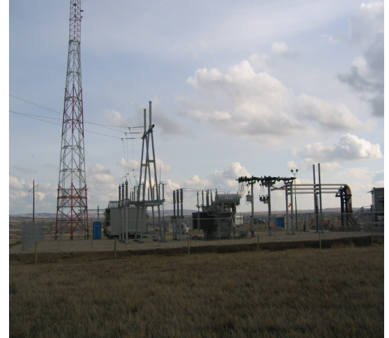
The proposed Twin Lakes Substation will be similar to the substation pictured above.
