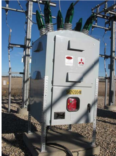
A typical 25 kV circuit breaker
