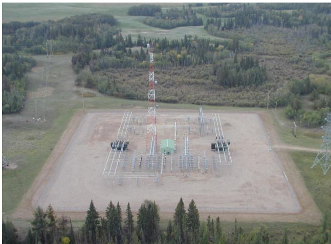
Above: the existing Deerland 13S substation
