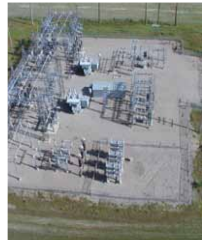
The proposed Harry Smith Substation will look similar to the one pictured here
