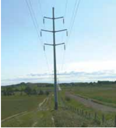
Above: 138 kV double circuit transmission structure
