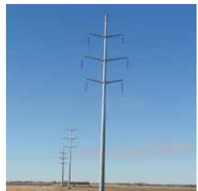
Above: Comparison of structures between the Heartland project and the Harry Smith (HS) project. (top to bottom) 500 kV lattice structure (Heartland); 240 kV H-Frame (HS); 138 kV steel monopoles (HS)
