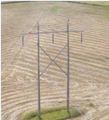
Above: 240 kV single circuit transmission structure
