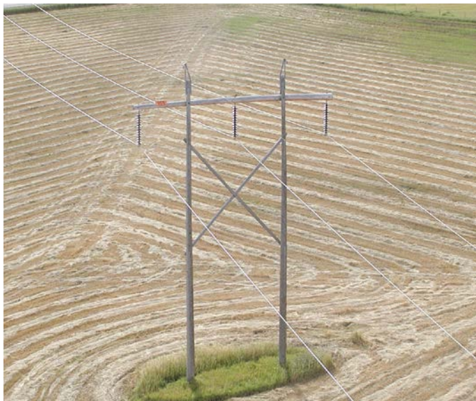
The structures on the proposed 1181L line will look mostly similar to the above, but the insulators may be configured differently.
