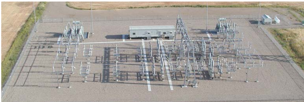
The existing Whitla Substation
