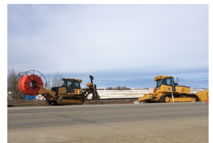
Above: Fibre optic cable being buried. You may see similar construction activities in your area.
