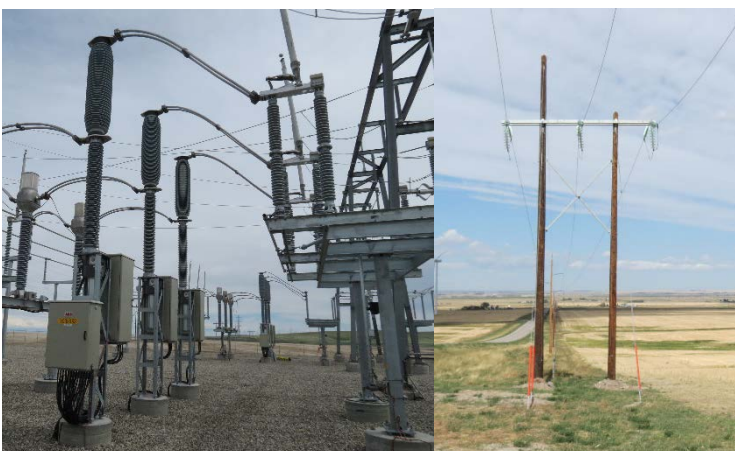
Left: A typical 240kV circuit breaker
