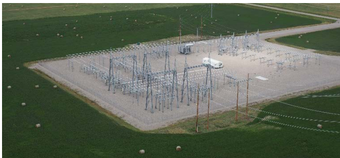
The existing Fidler Substation
