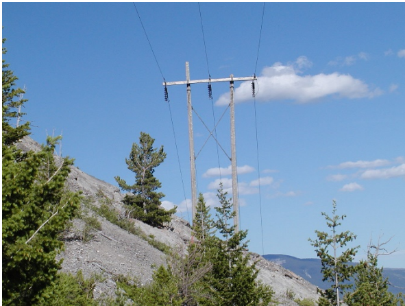
An existing H-frame structure on the 786L transmission line. The new structures will look similar, but will be taller.
