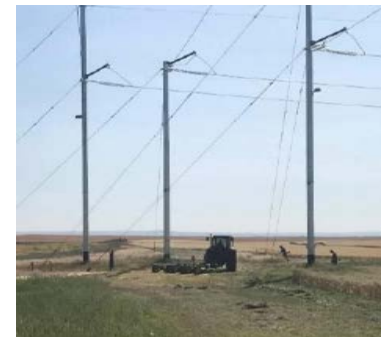
The three-pole dead end structure will look similar to the structure shown above.
