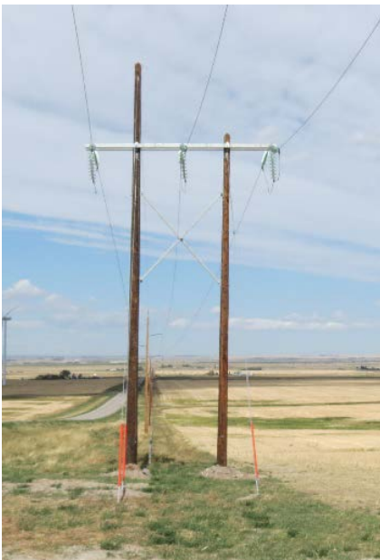
Above: A typical two-pole wood structure.
