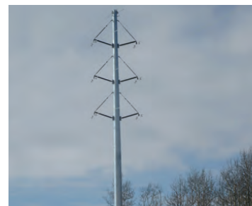
Top: Single circuit monopole Bottom: Double circuit monopole
