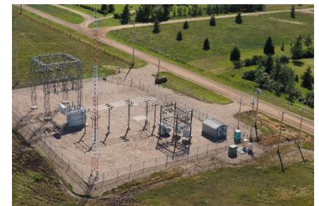
The existing 339S Duchess Substation
