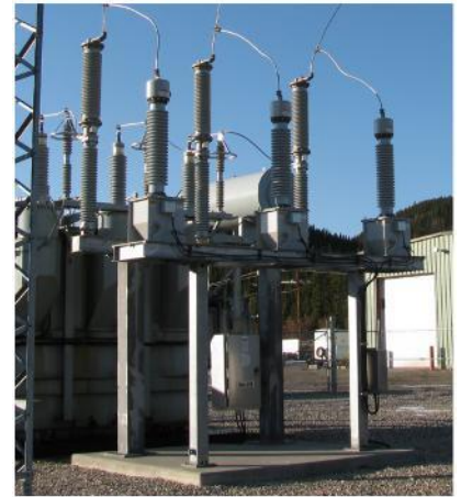
Above: a typical 138 kV circuit breaker
