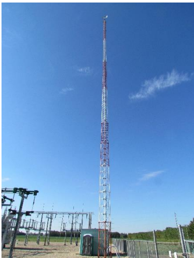
Below: The new telecommunication tower will be constructed within the Rattlesnake Ridge Substation, and will look similar to the one pictured below.
