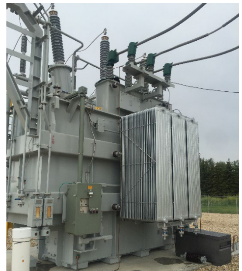
A 138 kV transformer
