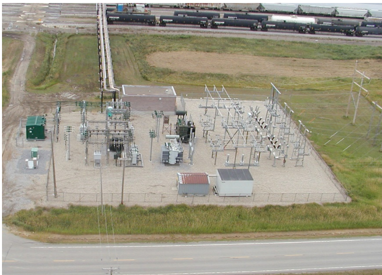
The existing Carseland Substation
