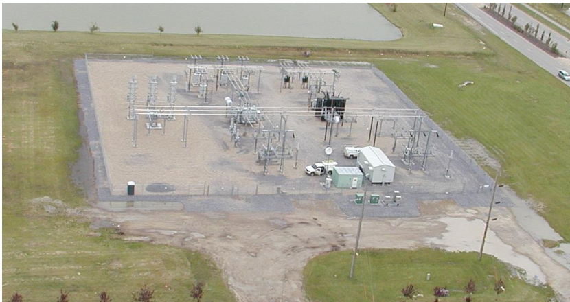
The East Airdrie Substation
