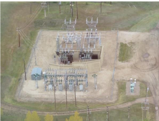
The Sherwood Park Substation
