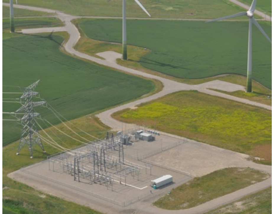
Existing Castle Rock Ridge Substation
