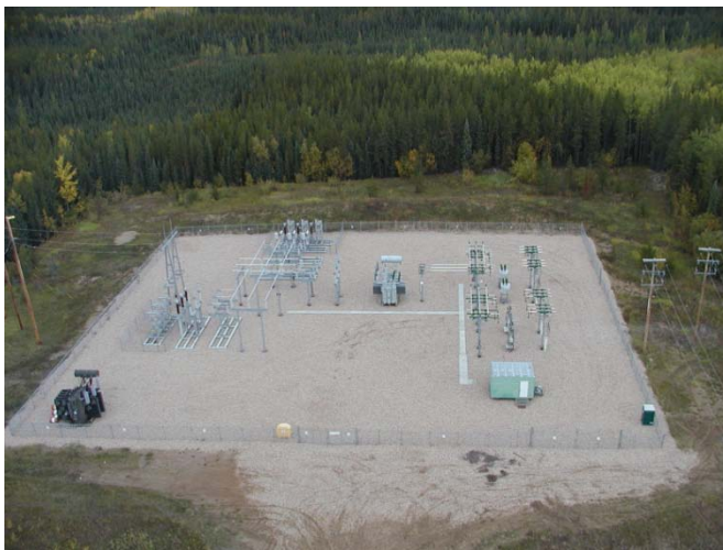
The proposed Grist Lake Substation will look similar to the one pictured here.
