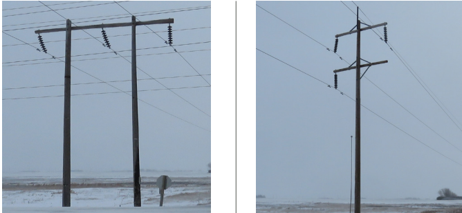
The existing H-Frame (left) and monopole (right) structures being proposed for removal. The new structures will look similar but will be taller.
