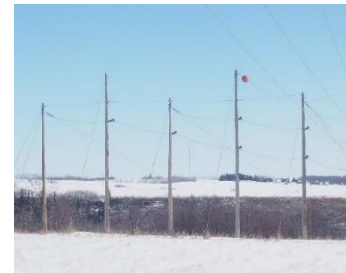
The existing six-pole clusters on the 759L transmission line look similar to the photo above
