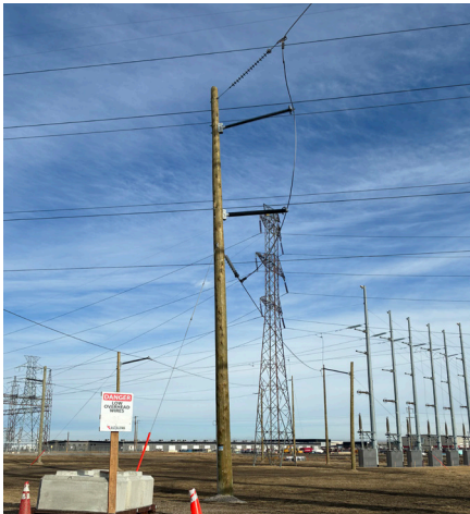
Left photo: The temporary bypass lines that have been installed to maintain reliable power during construction.
