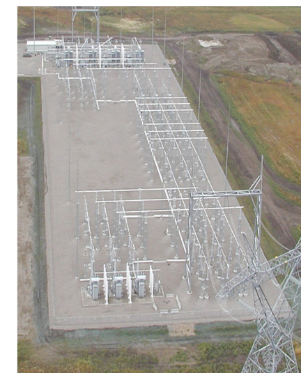
An aerial view of the Bennett Substation
