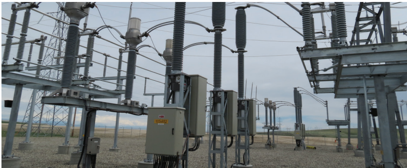
A typical 240 kV circuit breaker
