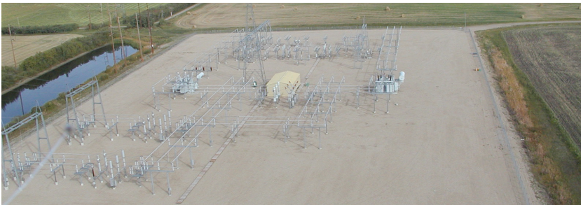
Existing Gaetz Substation
