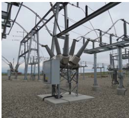
A typical 138 kV circuit breaker
