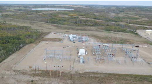
Existing Hansman Lake Substation
