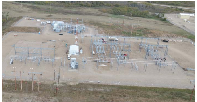
Existing Hansman Lake Substation
