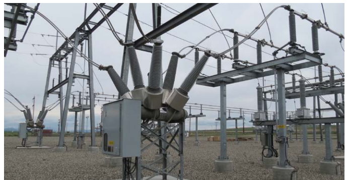
A typical 138 kV circuit breaker
