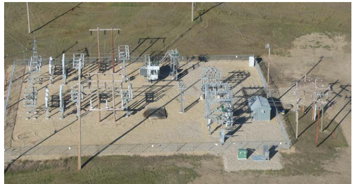
Existing Edgerton Substation
