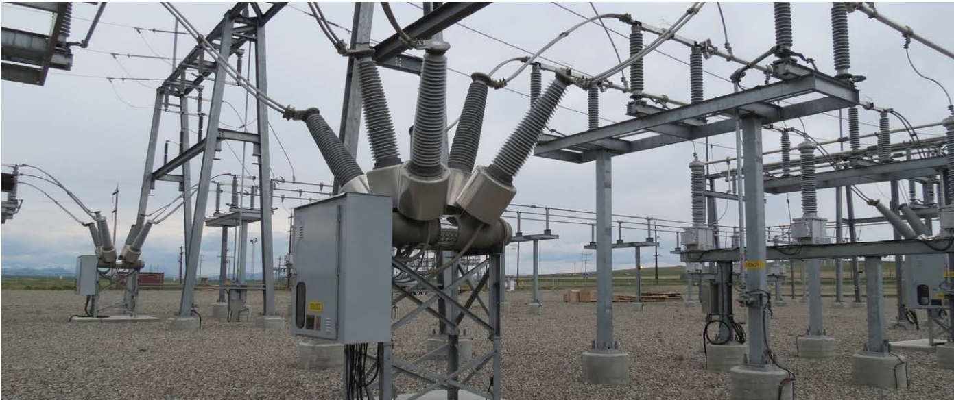
A typical 138 kV circuit breaker
