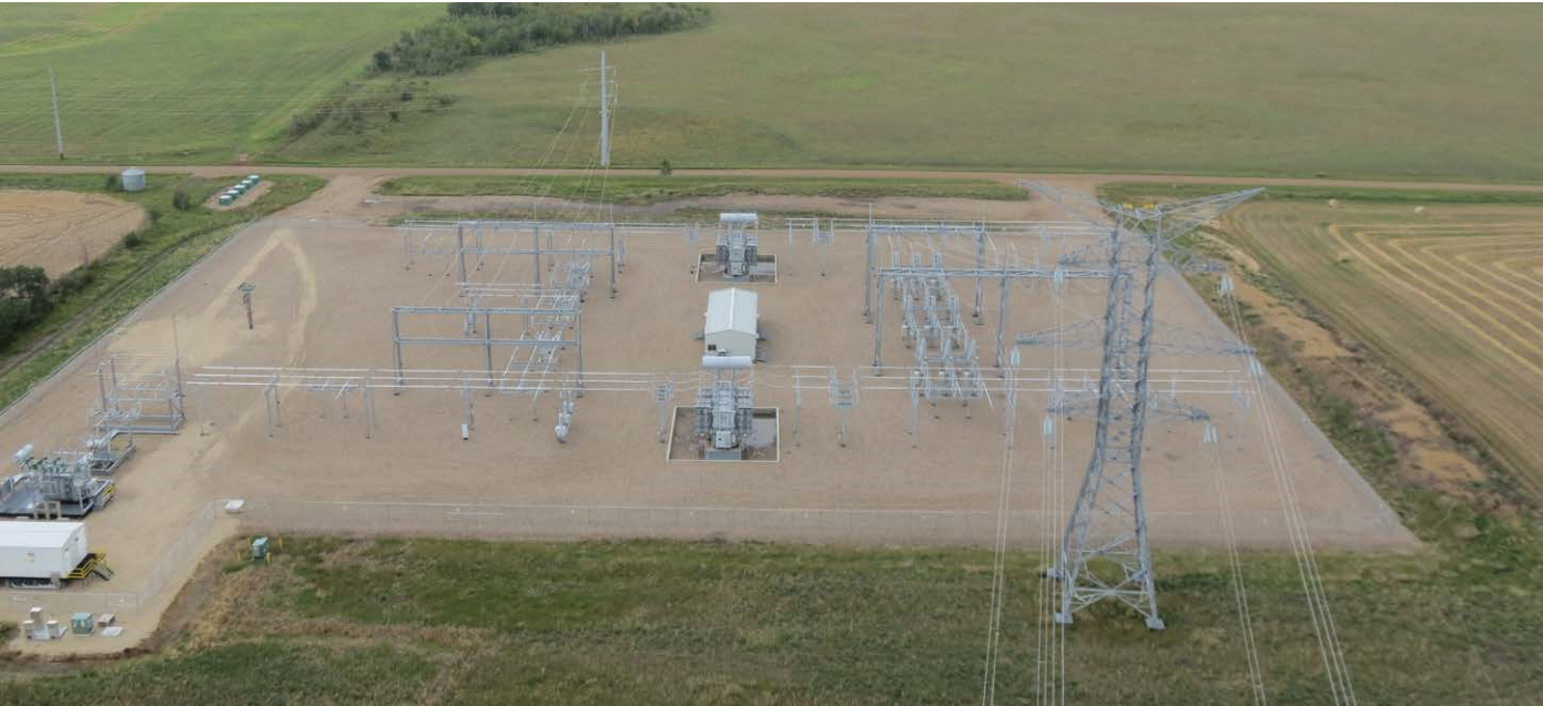
Existing Nilrem Substation
