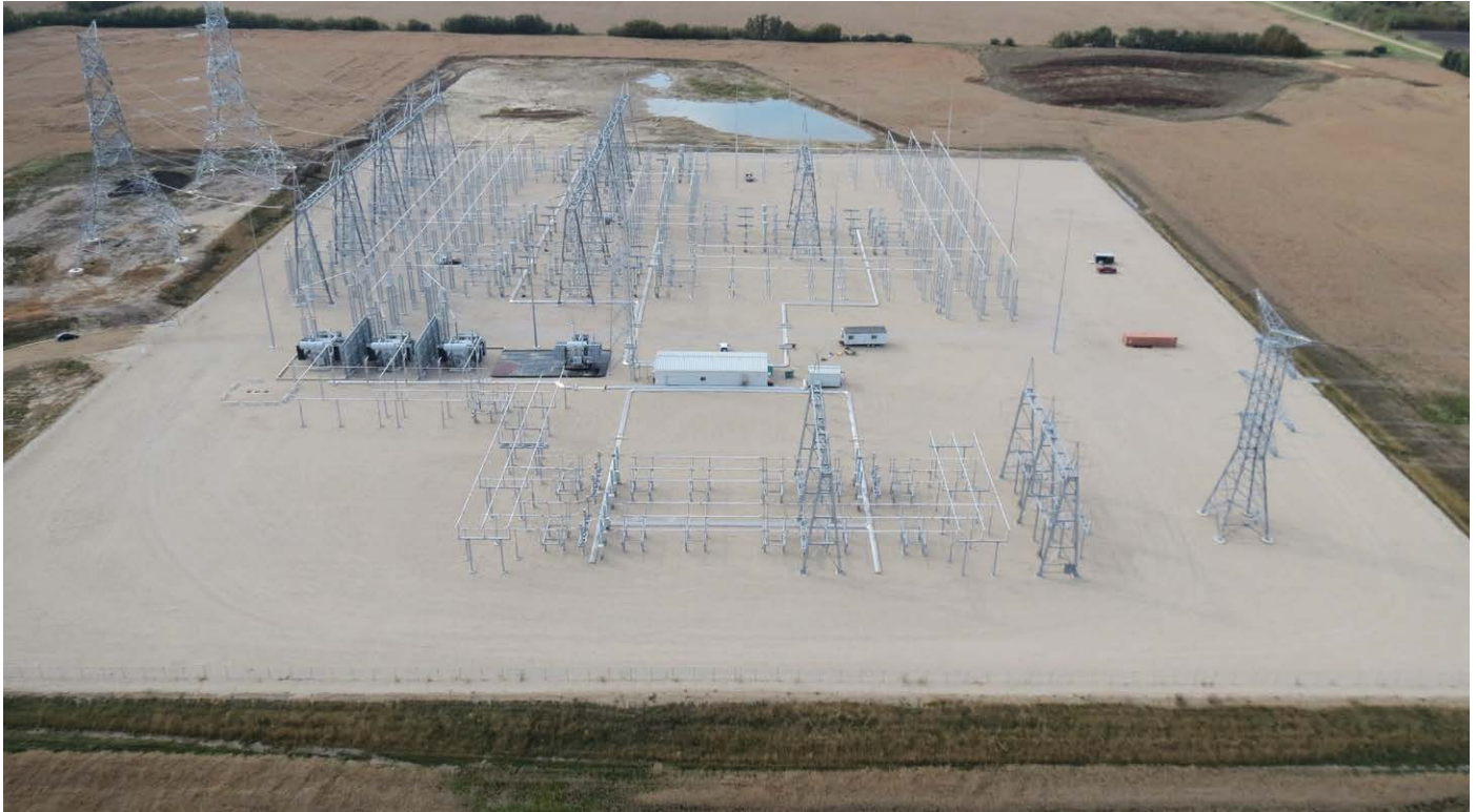
The Chapel Rock Substation will look similar to the one pictured here.
