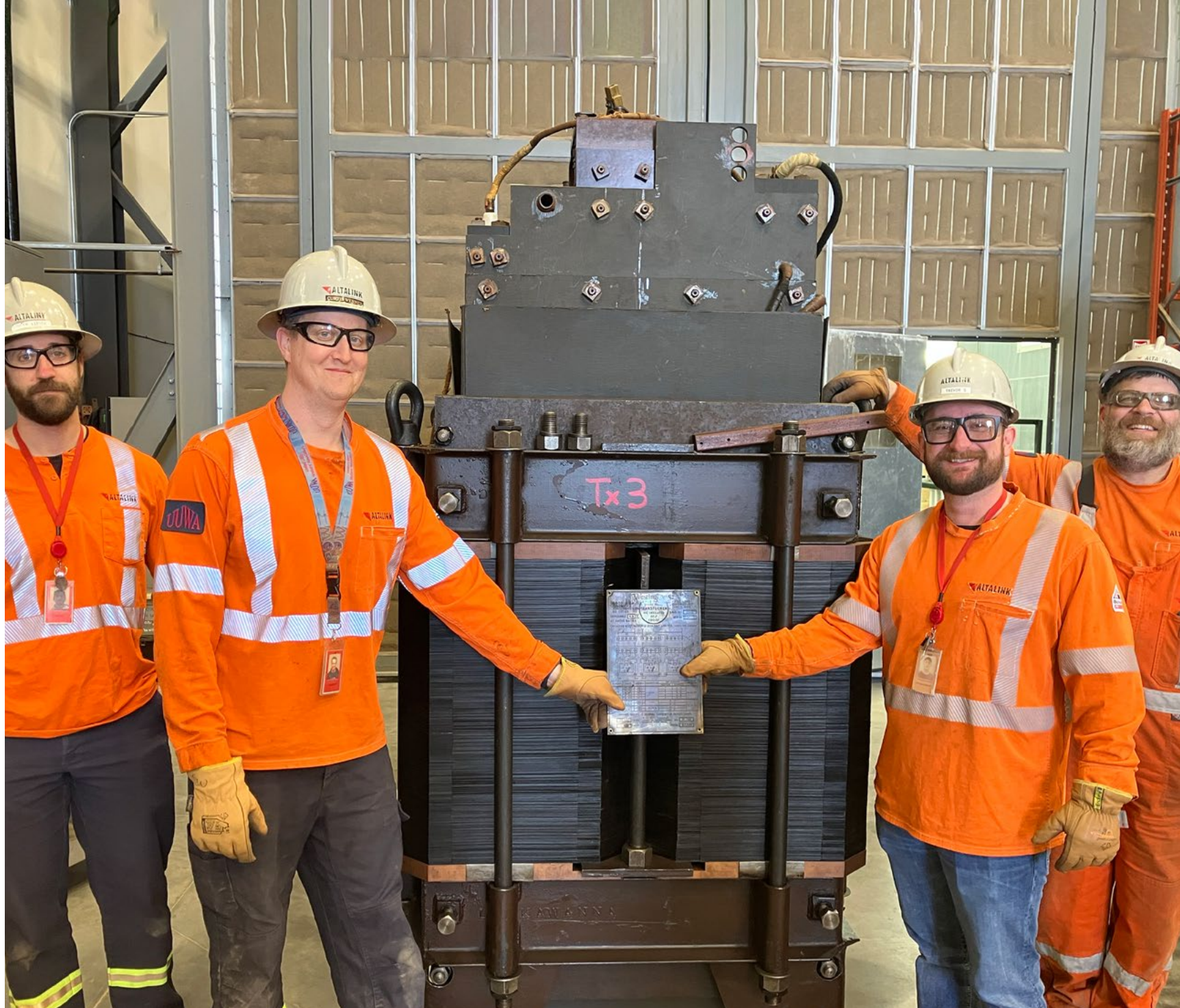
▲ AltaLink substation techs standing in front of a decommissioned transformer – one of the oldest in Alberta
