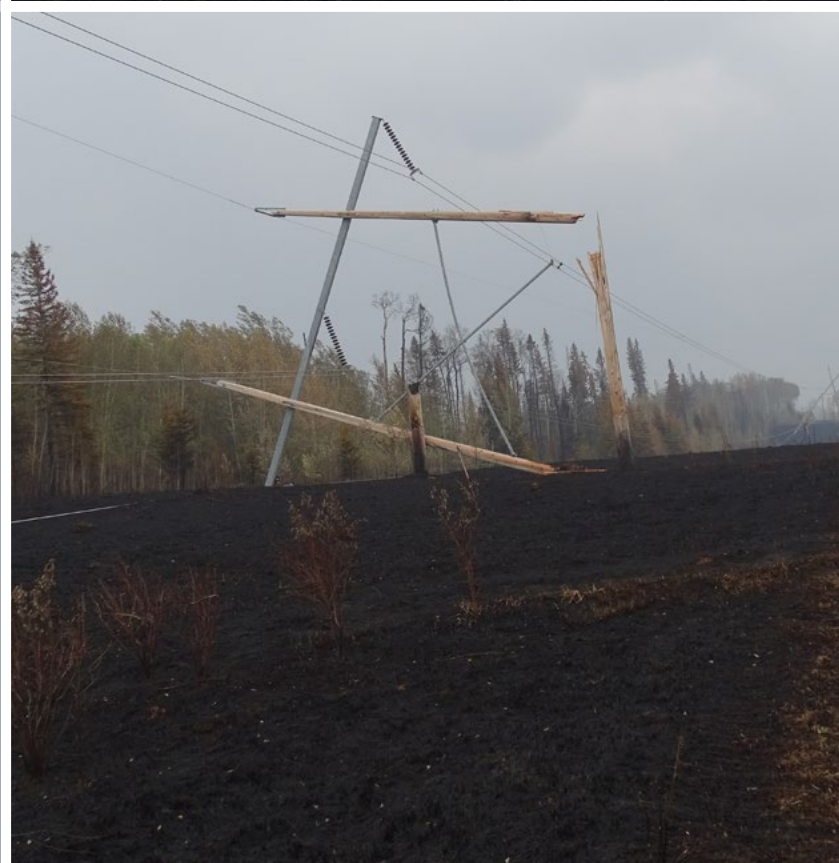
▲ Damaged transmission structures following the Lac La Biche wildfire
