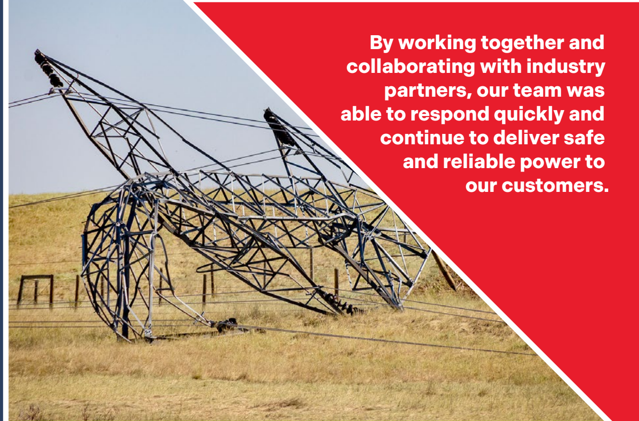
▲ Damaged transmission structures following the tornado in the Brooks area
