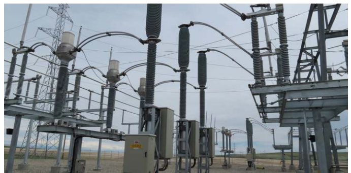
A typical 240 kV circuit breaker
