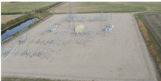
Existing Gaetz Substation
