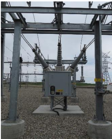
A 240 kV circuit breaker
