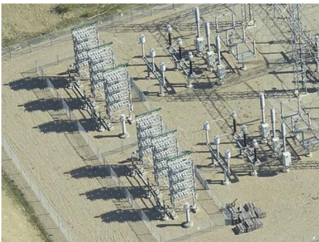
A capacitor bank
