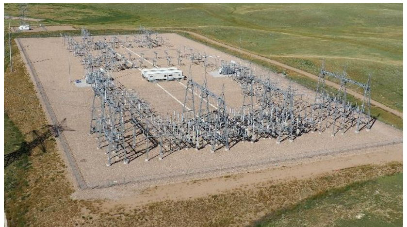
The Bowmanton Substation
