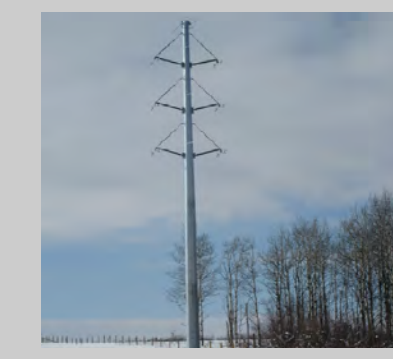
Double Circuit Monopole
