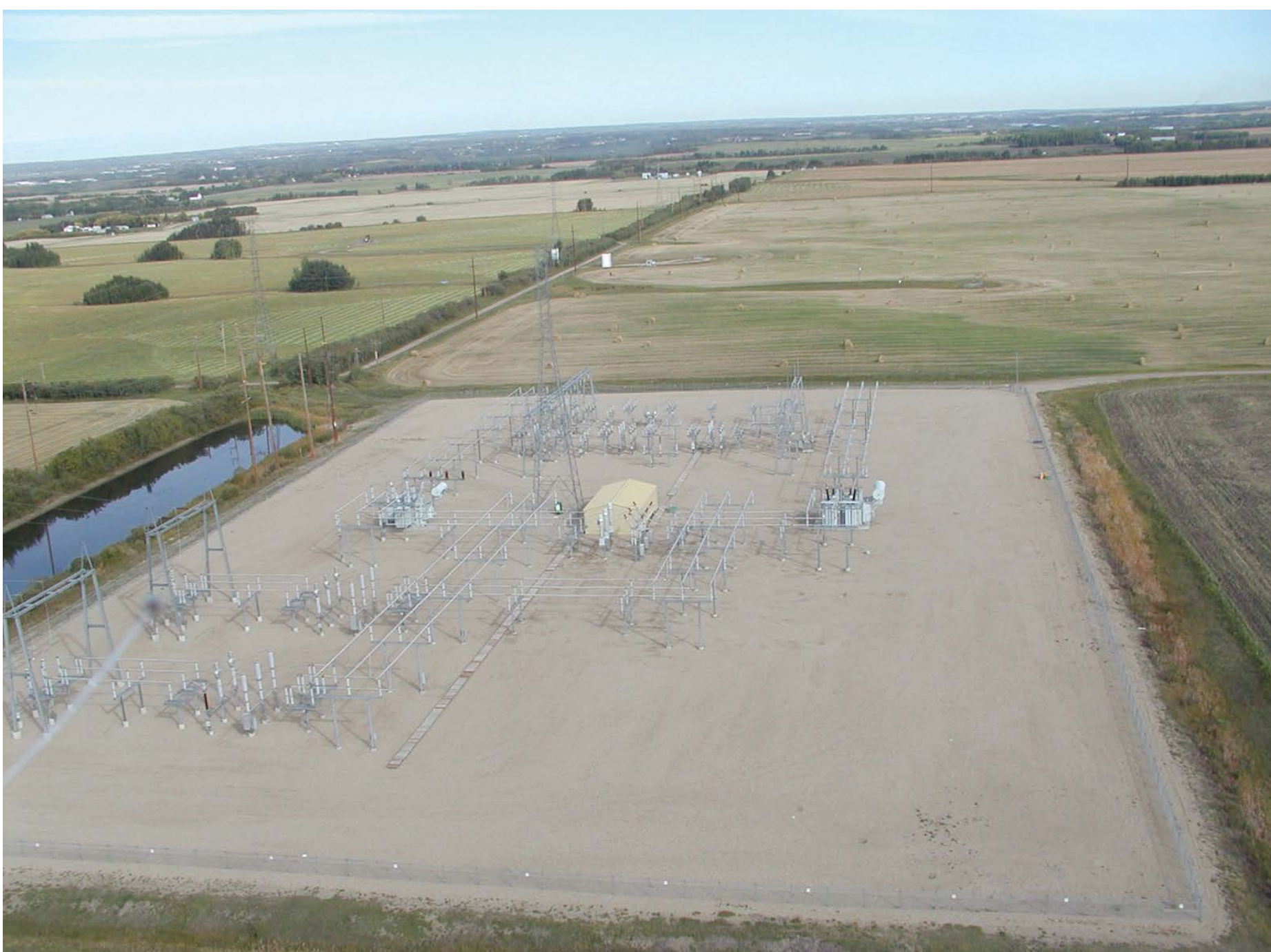
Existing Gaetz Substation
