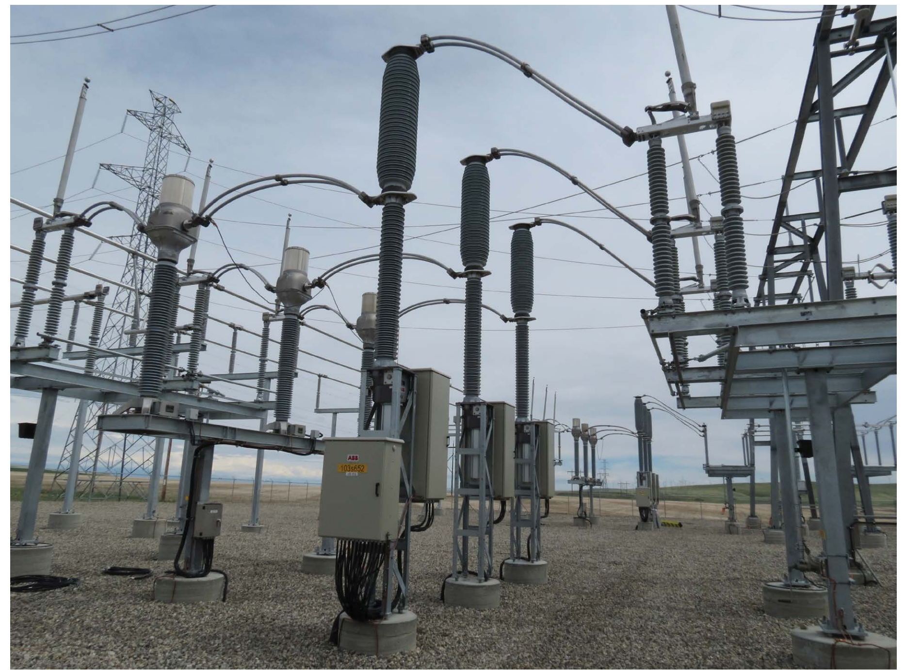
A typical 240 kV circuit breaker
