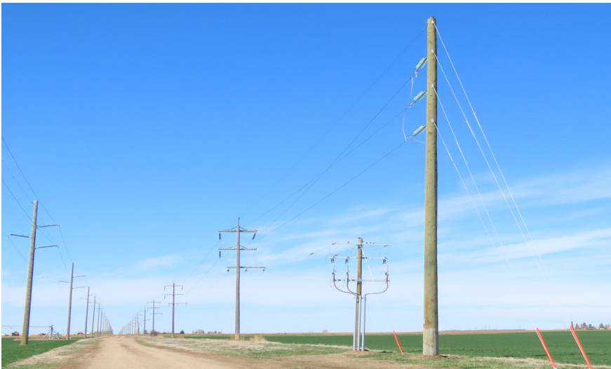
Above: The existing D610L transmission line is shown on the right.
