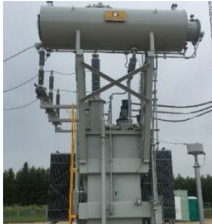
The new transformer will look similar to the picture above
