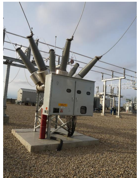
138 kV circuit breaker
