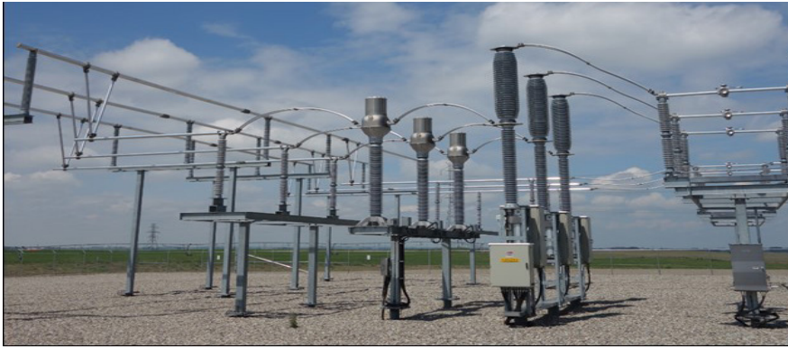
The new circuit breaker will look similar to the picture above
