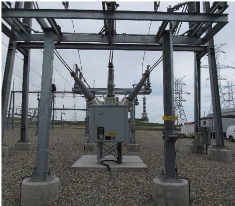
Above: A typical 138 kV circuit breaker
