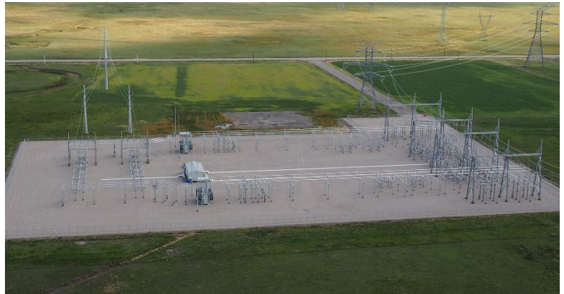
Above: The existing Foothills Substation
