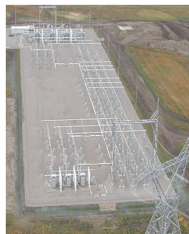
An aerial view of the Bennett Substation
