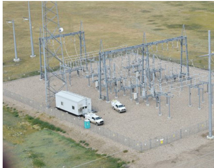
This is an example of a similar switching station.
