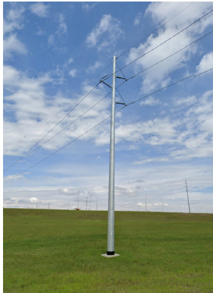
Above: Steel monopole structures will look similar to the one shown in the photo
