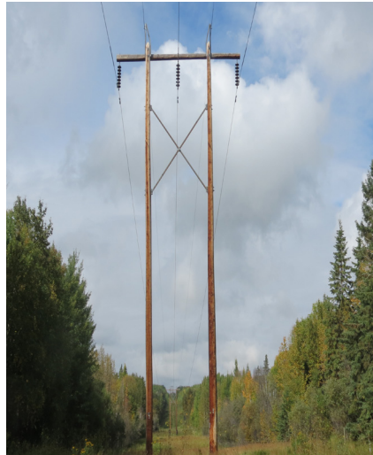
Above: Wood H-frame structures will look similar to the one shown in the photo
