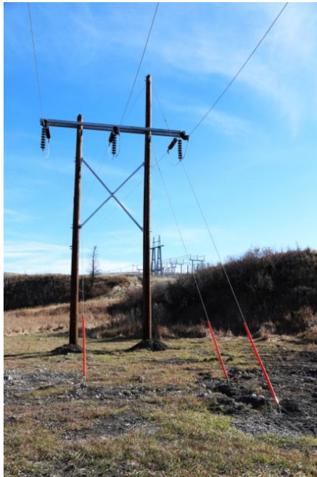
The proposed structure on the 164AL line will look similar to the structure above.
