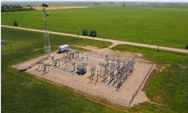
Above: The existing Vauxhall Substation
