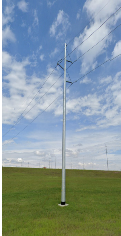
Above: Steel monopole structures will look similar to the one shown in the photo
