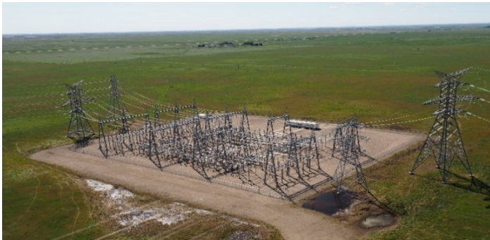
Above: The existing Cassils Substation
