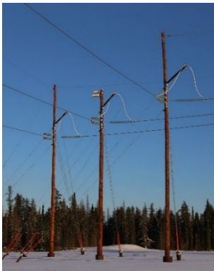
Angle structures with guy wires will look similar to the three-pole structure shown above and may be wood or steel.
