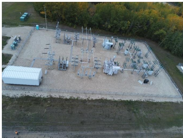
The St. Albert Substation
